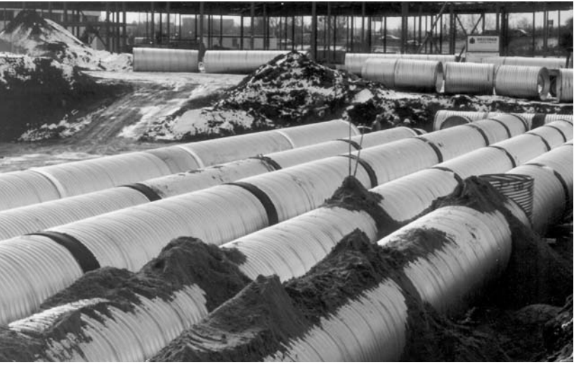
Stormwater detention system.
