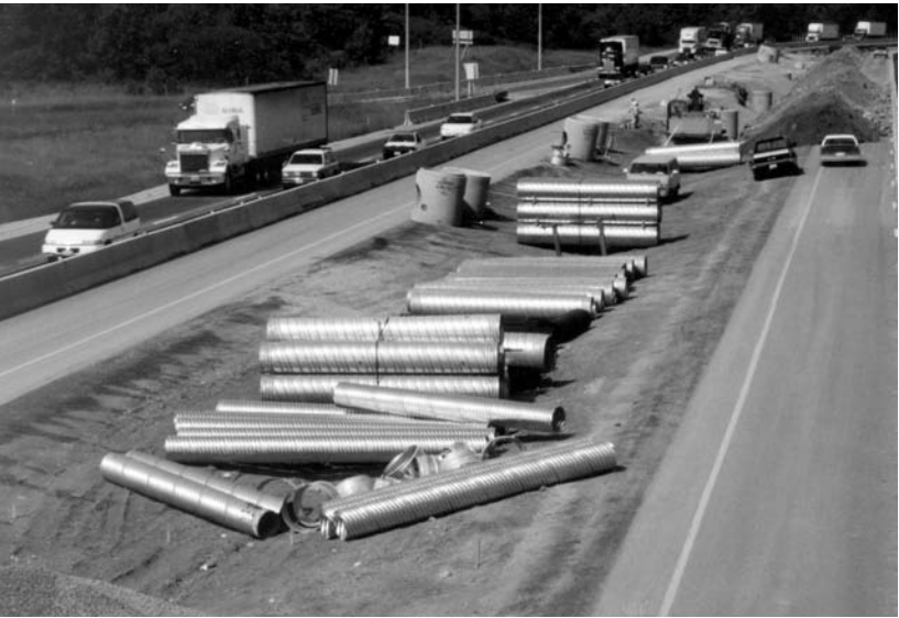
Highway 401 in Ontario using spiral rib steel pipe and corrugated steel pipe for median drainage.
