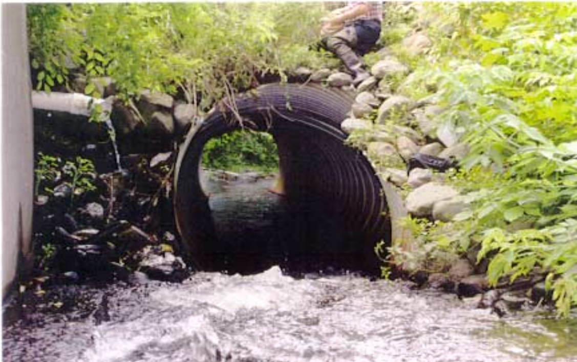
Figure 7. Culvert at Dexter, Maine, experiencing high-velocity flow.
