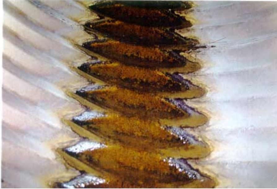
Figure 6. Aluminized Type 2 culvert after 5.5 years exposed to runoff with a pH of 2.5 to 3.5 (not from this study).
