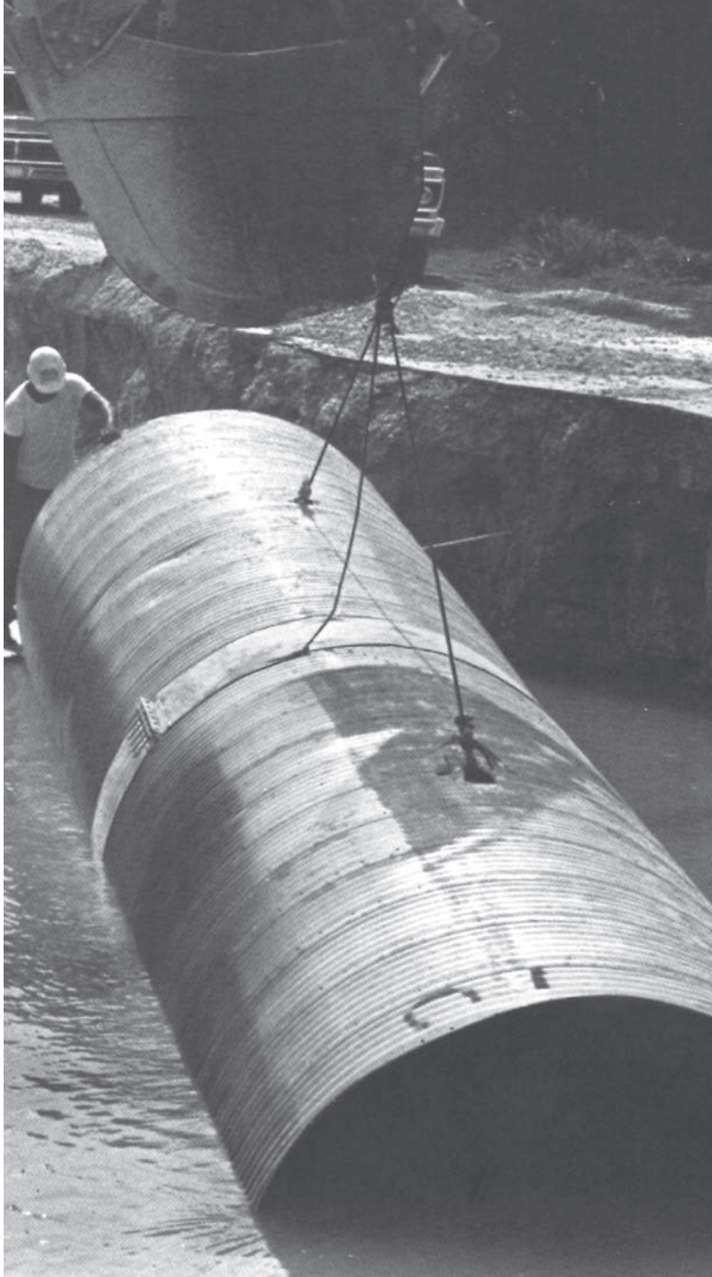
Two 6m joints of fully perforated pipe banded together for ease of installation.
