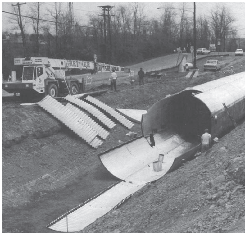
100 m of 3800 mm diameter, 2.8 mm structural plate pipe with gasketed seams used as an underground detention chamber collecting runoff from a shopping center.
