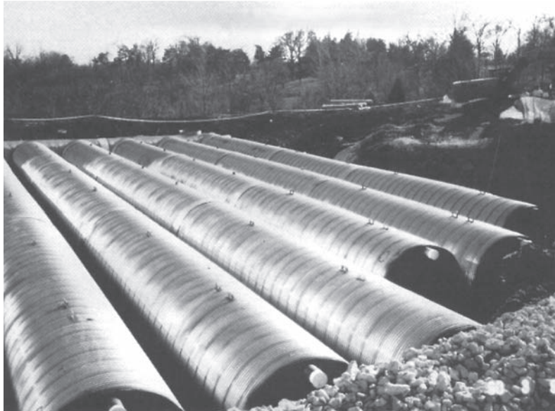
2700mm, diameter, 2mm, 76 x 25 CSP used as an underground detention chamber. The outlet control structure is located at the opposite end and to the right of those pipe.
