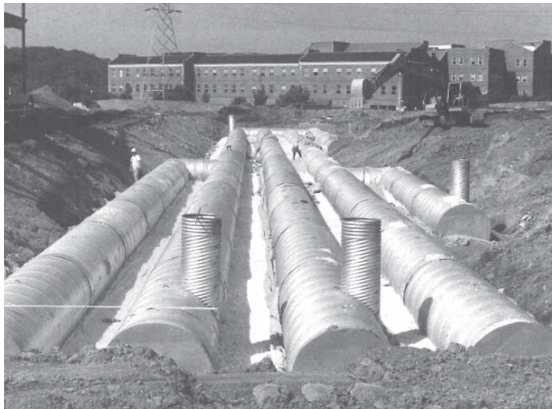
An example of a combination underground detention chamber and recharge system. Five lines of 1800 mm diameter corrugated steel pipe with 150 mm slots in the invert.
