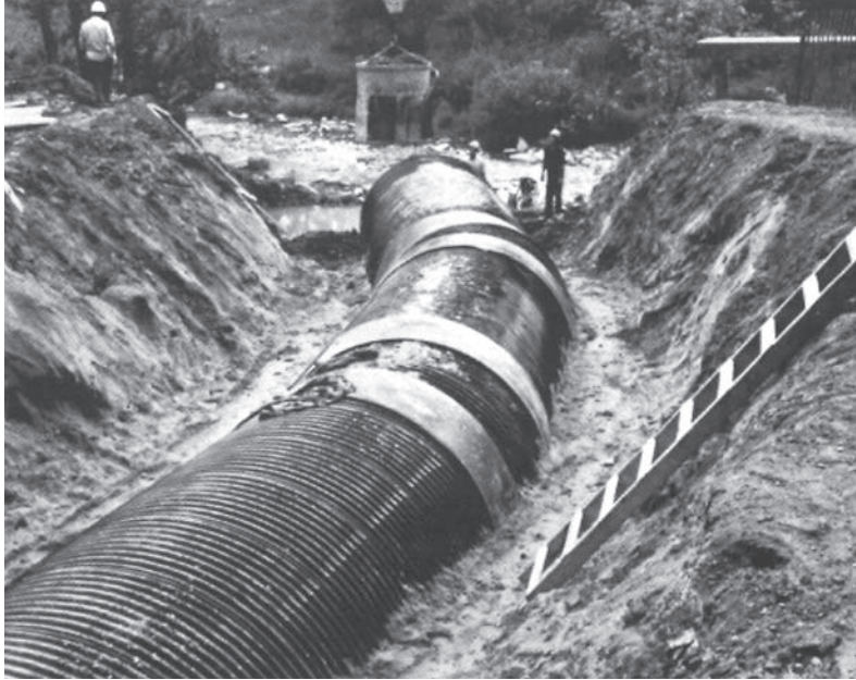
Outfall for 2200mm CSP storm sewer. Entire line averaged 5% grade, which is suited to choice of steel
