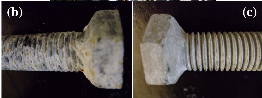
FIGURE 4 (a) Example of staining in the obvert of a structure coated with the thermoplastic polymer system. (b) Galvanized bolt following removal from test chamber compared to (c) duplex coated bolt at three times the exposure time.
