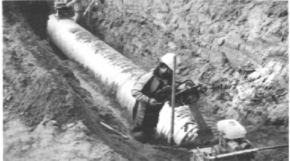
Markus Construction crew compacts granular backfill during the installation of Ultra Flo Pipe
