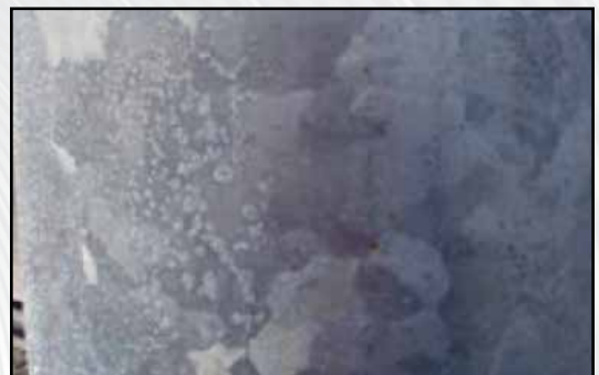
FIGURE 1 - WET STORAGE STAIN
