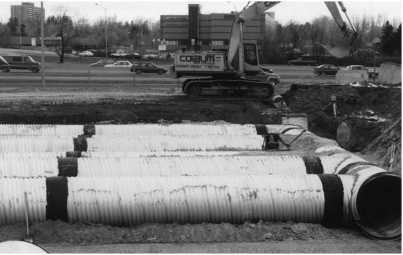
Joints wrapped with geotextile to prevent migration of fines into the pipes.
