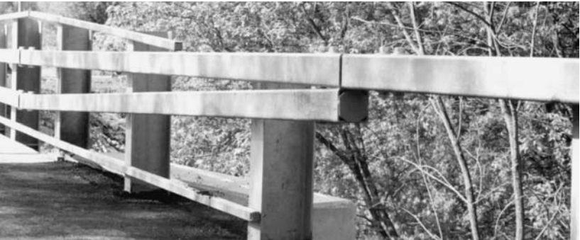
Transition from bridge rail to box-beam guiderail.
